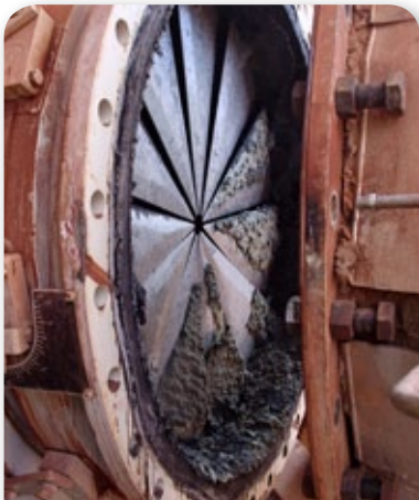
Blower condition - after opening on site
